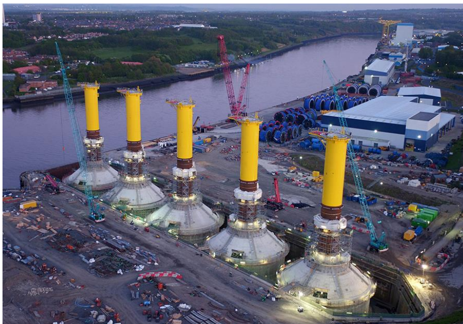
Figure 15 BAM Nuttall concrete GBFs for Blyth windfarm, using steel shafts (source: BAM).
