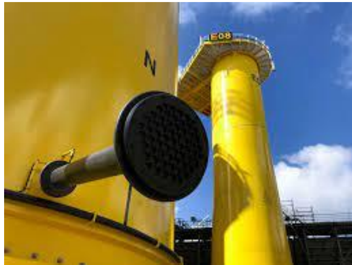
Figure 13 ICCP anode fitted on a transition piece (source: Corrosion.nl).
