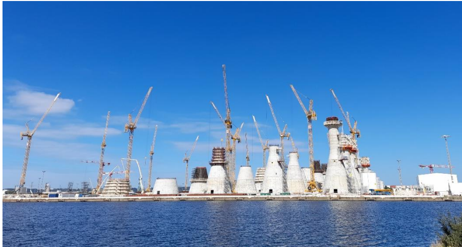
Figure 17 Industrialised construction of GBFs by Bouygues Travaux Publics at Le Havre for Fécamp (source: Bouygues).
