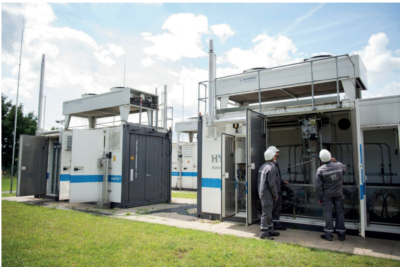
Figuur 23: AEL Elektrolyse (Hydrogenics) Falkenhagen Germany
