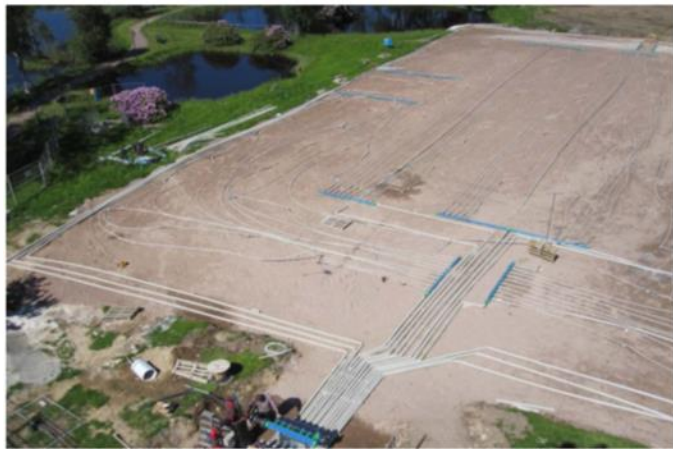
BTES system from Emmaboda Sweden
