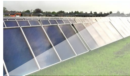
Solar district heating
