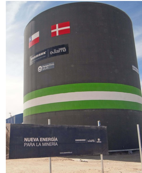
Picture from a project of F.W. Rørteknik of a 4'500 m 3 TTES in Chile. See: https://www.fw.dk/references/4500-m3-heat-storage-tank-chile/ for more information
