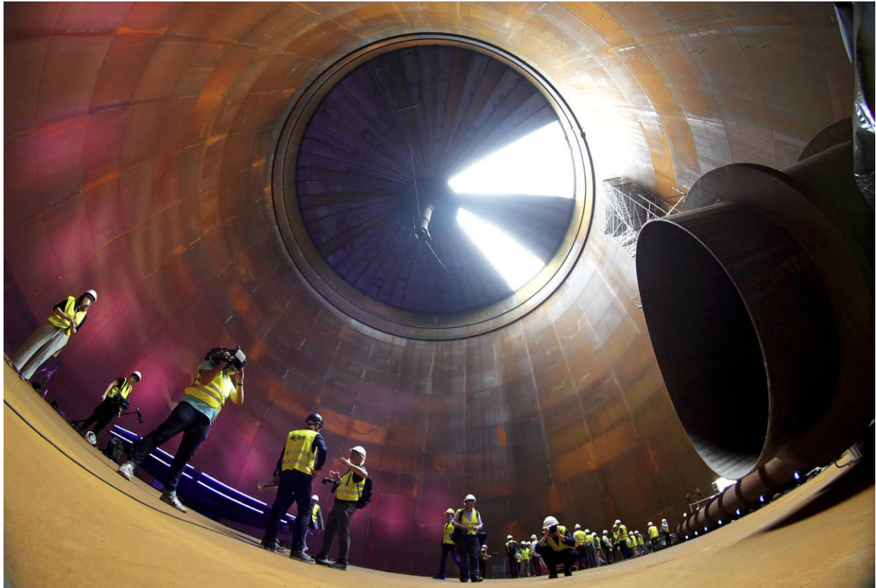
Figure 2: Inside of large 55.000 m 3 , 200 MW tank for Vattenfall heating network in Berlin
